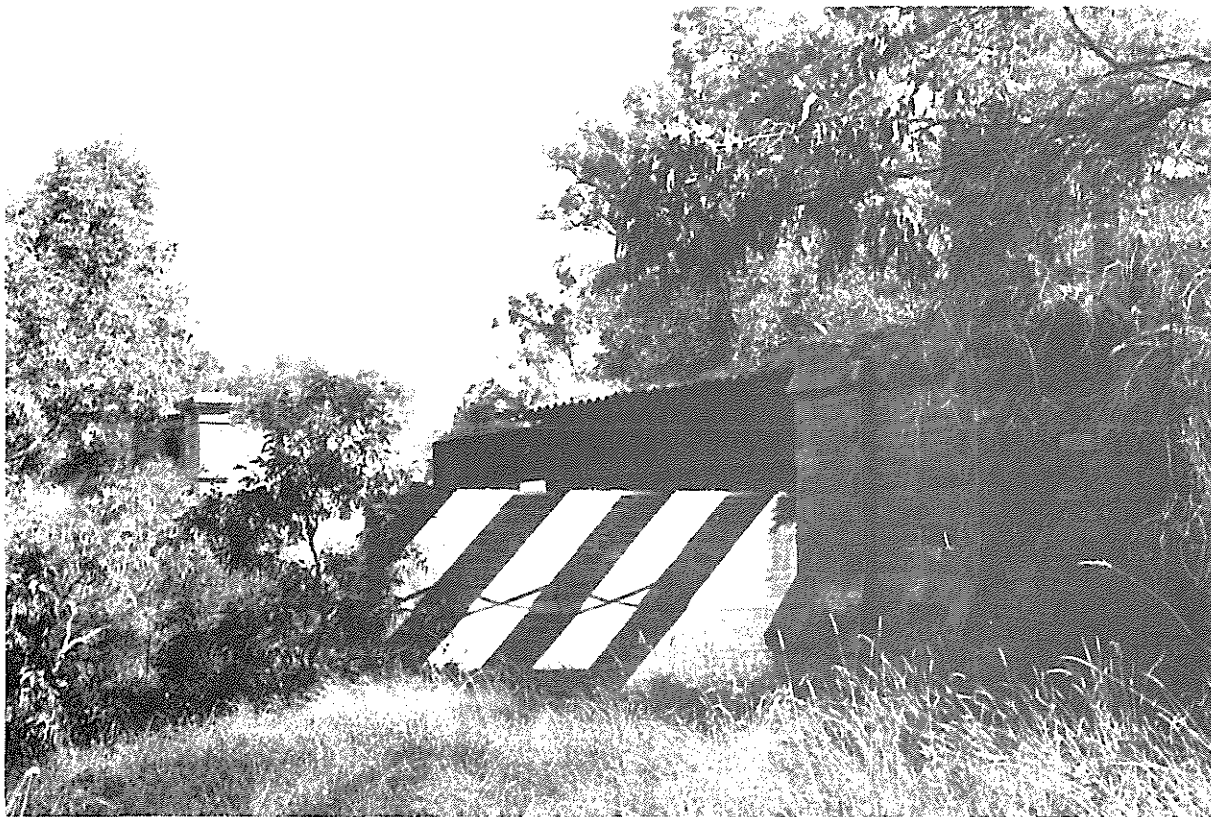
B.7.1.4 Ruined Bridge, Goolwa Road, Ashbourne
